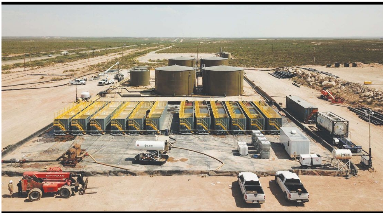
Solaris' Lobo Ranch water recycling plant came online in July. (Source: Solaris Water Midstream)
